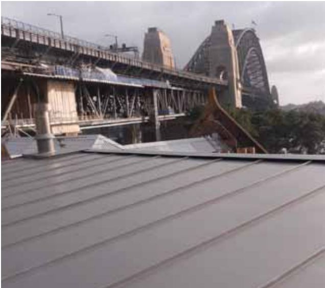
Commercial Building, The Rocks, Sydney, Installed by Roofing Group VMZINC Quartz-zinc, Double Lock Standing Seam roofing
